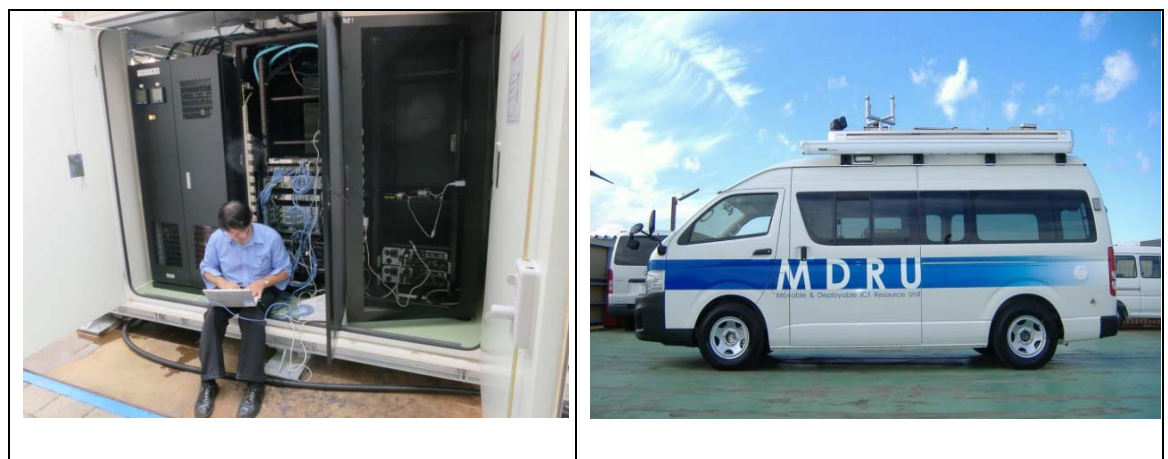
Figure 5.3 Components Inside MDRU & Vehicle Equipped with MDRU (ITU, 2015)
