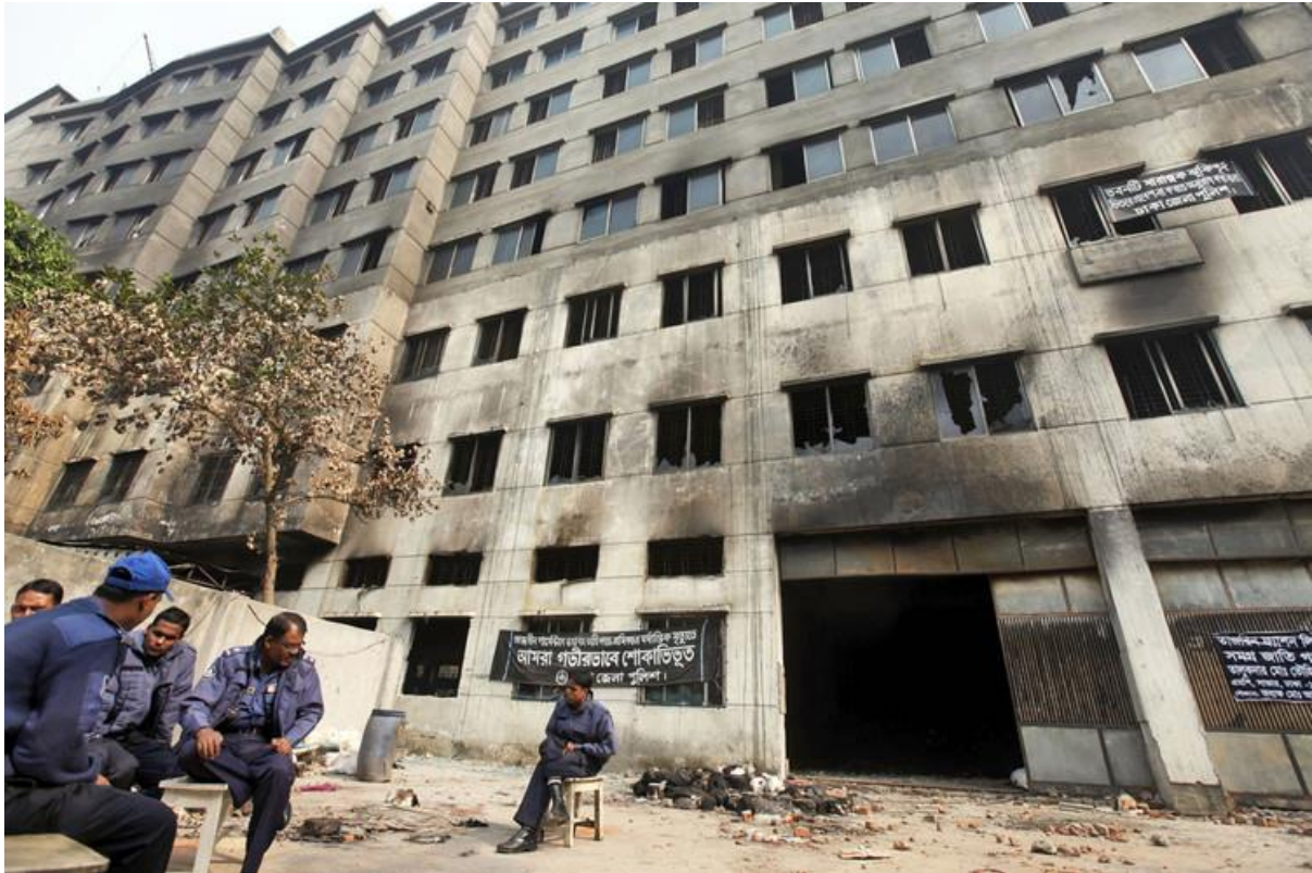
Figure 3 : Tazreen Fashion ltd. status after the fire hazard.
