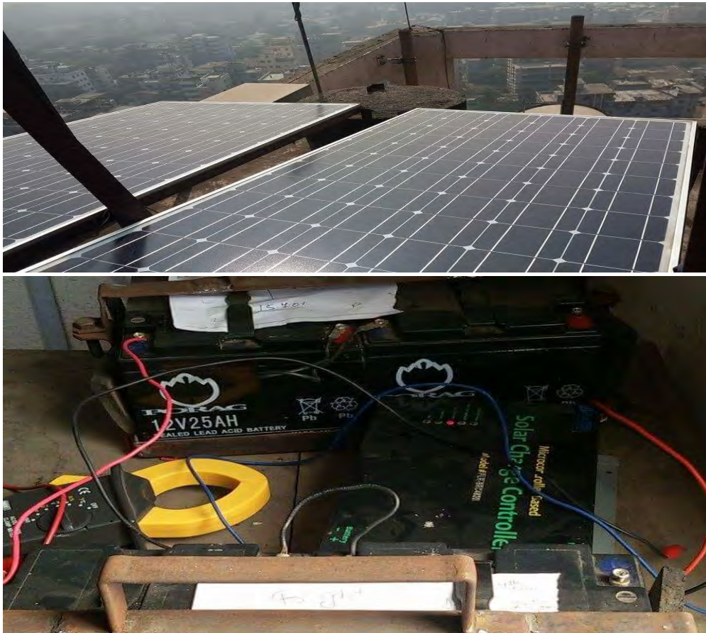
Fig 5.1 SBCS on the rooftop of BRAC university building 2
