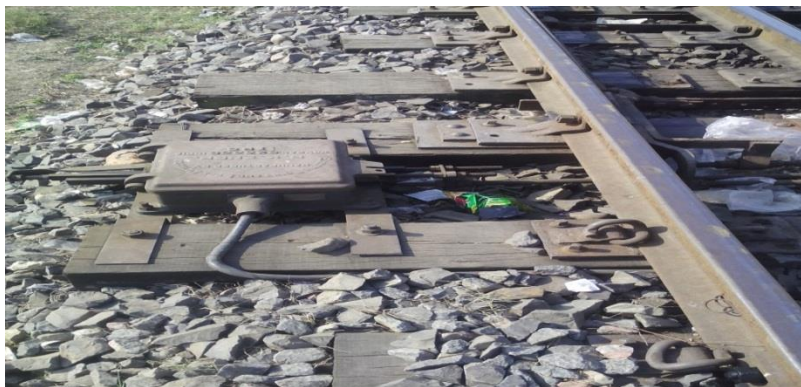
Fig 1.3: Mechanical Control box containing Electronic (Solid State) Interlocking and Relay based Interlocking
