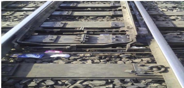
Fig 1.2: Moveable Rail Track
