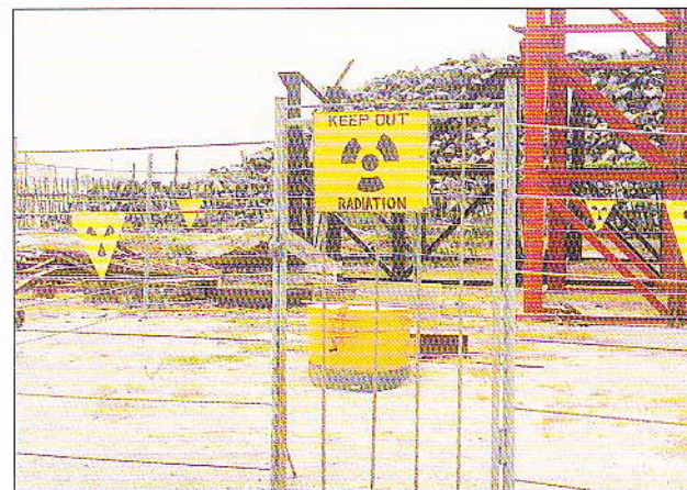
Typical Radio Isotope storage pit at site
