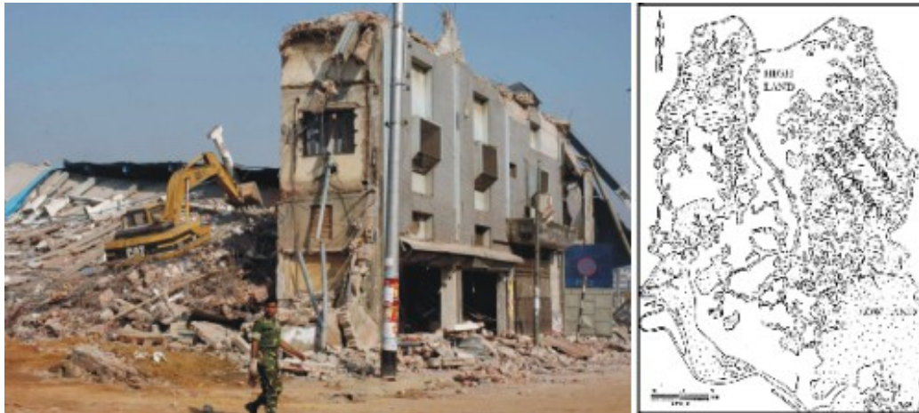
Figure 2.7: The collapsed building in Mohakhali, 2006 (Source: http://archive.thedailystar.net/2006/03/04/d603041501115.htm )
