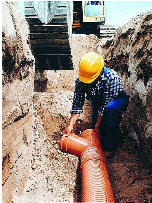
PVC pipe for sewerage line
