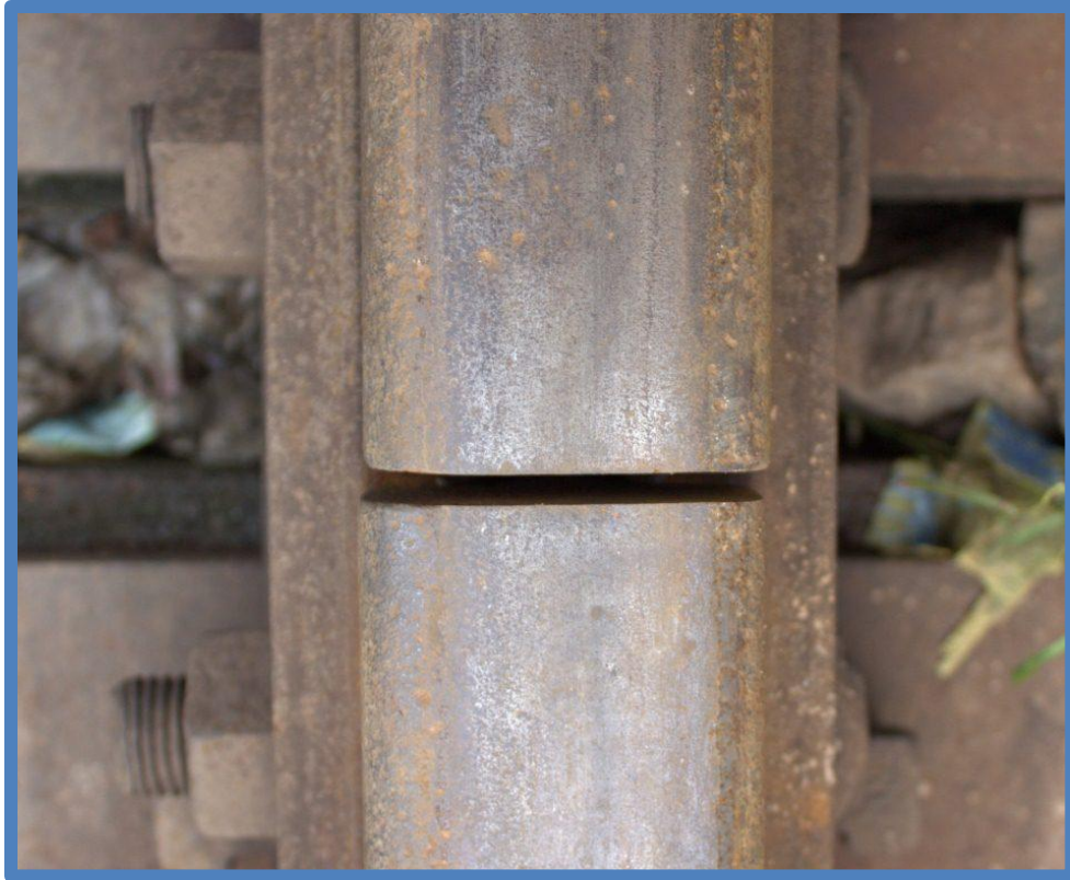
FIG: 1.1 Expansion joint gaps
