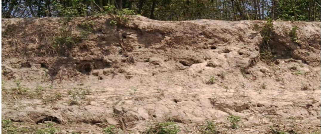
Figure 4.10 Present Erosion Situation at Sherkandi
