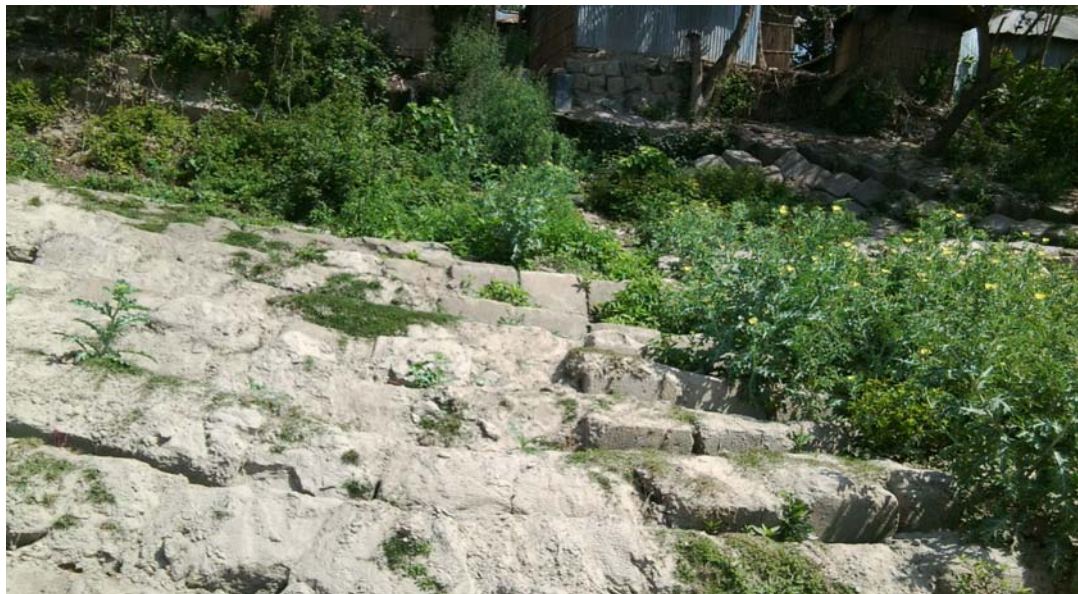
Figure 4.11 Houses at risk (Revetment near Kumarkhali M. N. High School)
