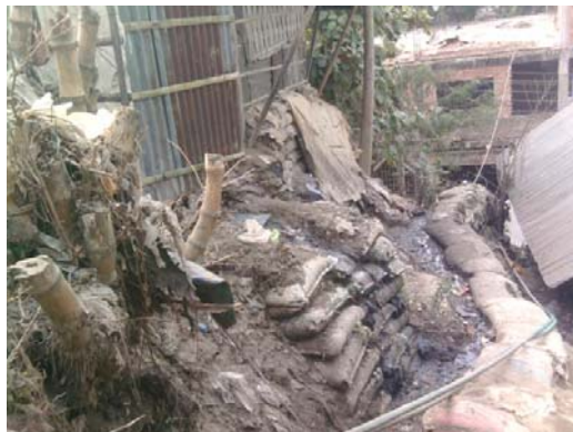
Fig: 4.16 Poor Drainage Source: Author, 2013
