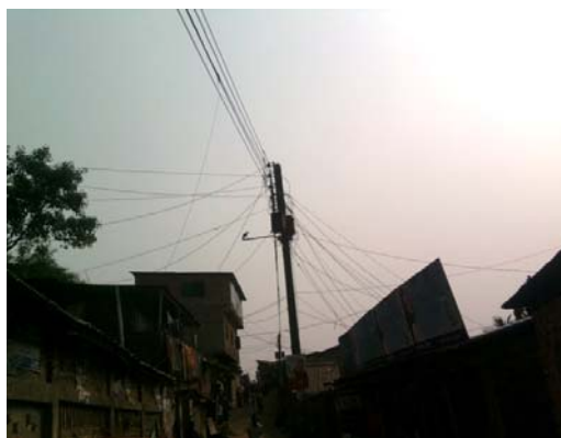
Fig: 4.14 Multiple illegal connections from a single pole
