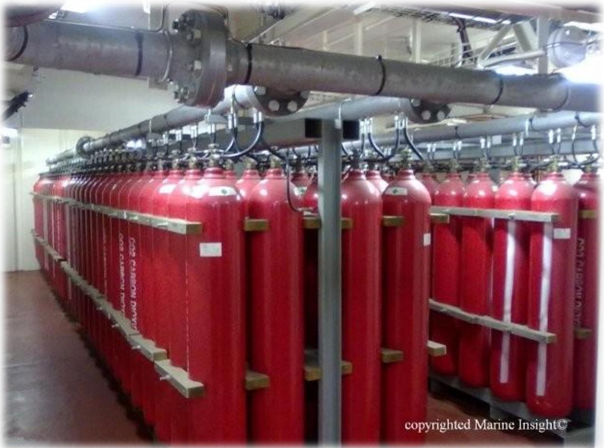
fig: CO2 tanks of ships' engine room.
