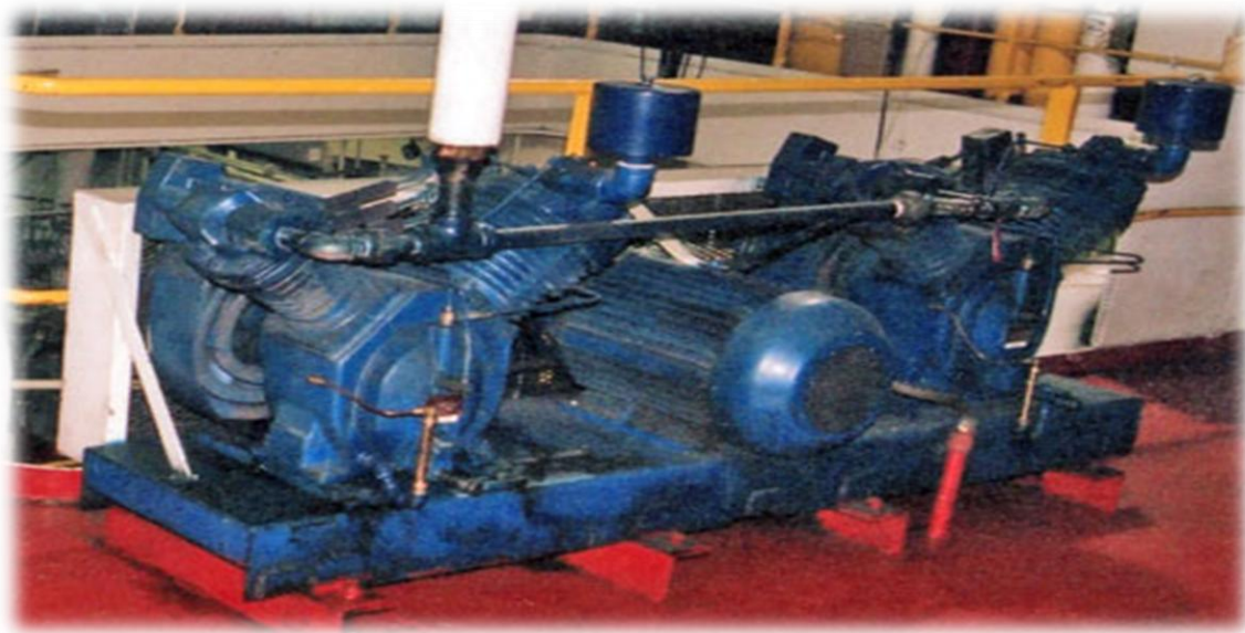
fig: Compressor of ships' engine room.
