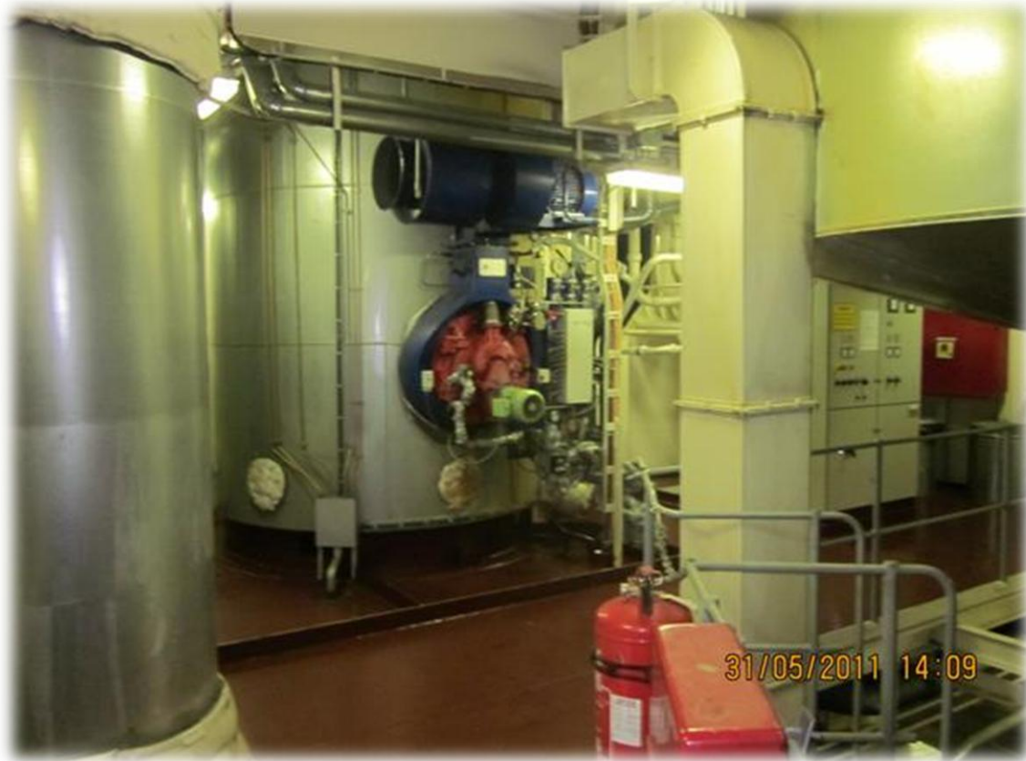
fig: Boiler of ships' engine room.
