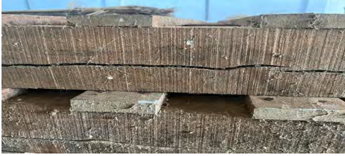
Fig 32: A crack is identified after supplying of dunnage to the Department of Food due to no-compliance of quality check.
