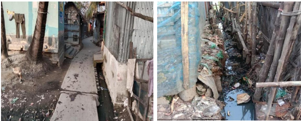
Figure 20: Poor Drainage system around the houses of Block B of railway slum area
