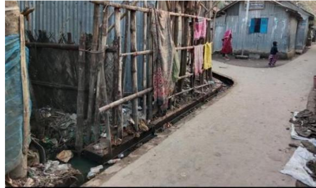
B: Poor drainage system of the slum
