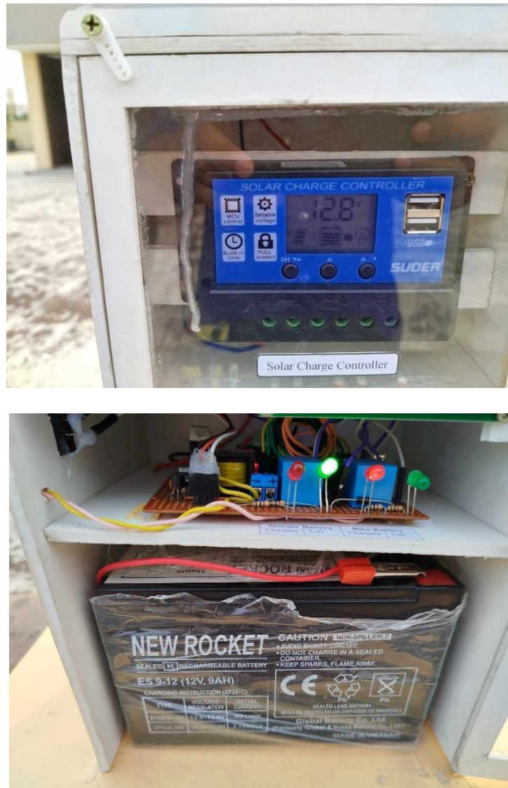
Fig. 5.2.3. Solar power generation and station battery
