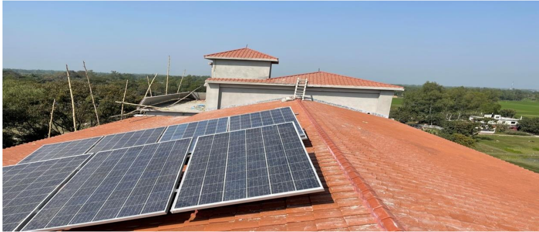
Fig6: Solar energy using in roof top in newly constructed educational building
