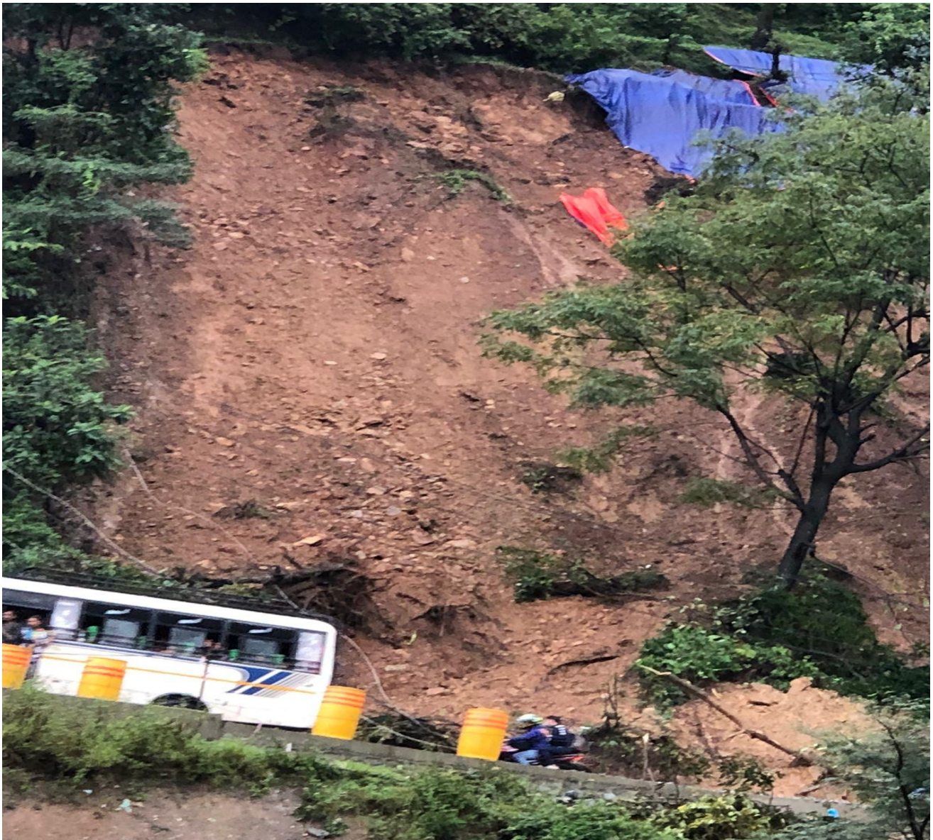
Figure 8 highway road erosion, (Author, 2022)
