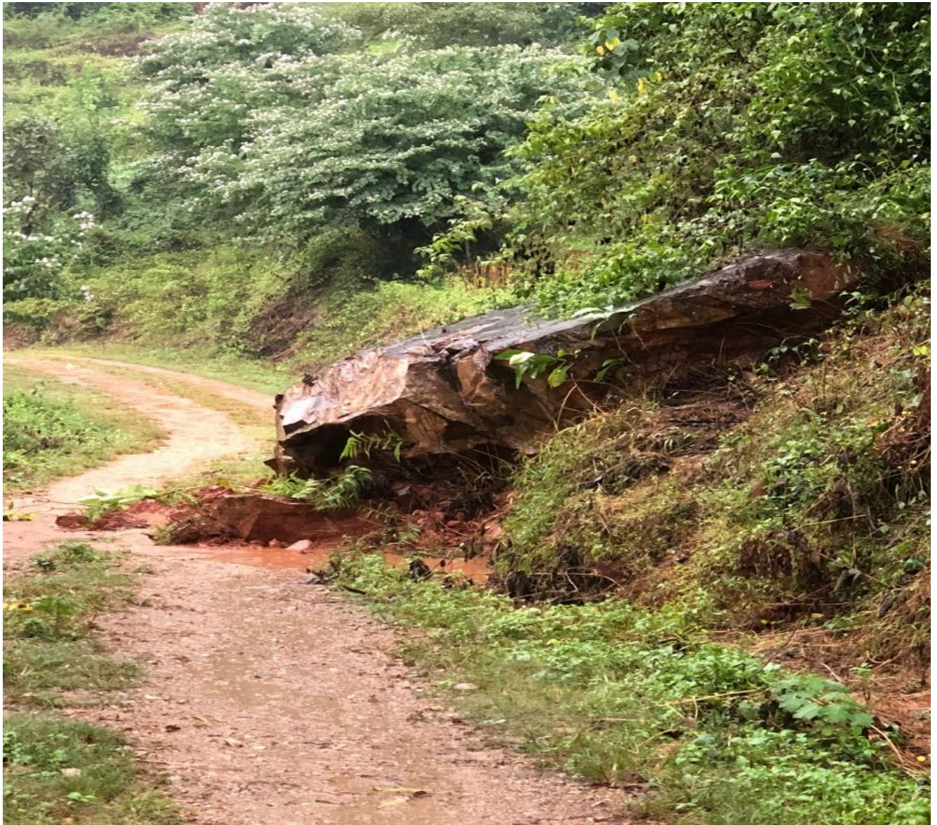
Figure 9 fallen rock after continuous rainfall, (Author, 2022)
