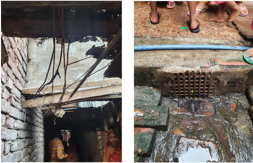
Fig 03: Exposed electrical wire and gas pipe in slum (Author, 2022)
