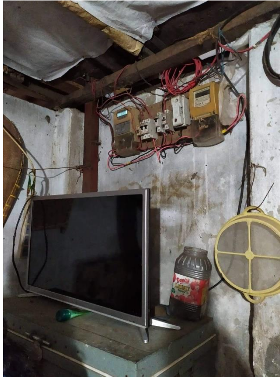
Fig 33: Electric connection drawn from outside to one of the rooms without professional supervision (Site survey, 2021)
