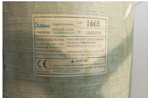
Figure -18: Pressure Vessel
