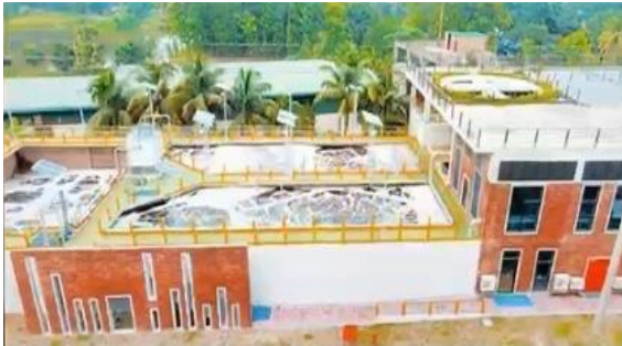
Figure 15: The New Effluents Treatment Unit(ETP),
