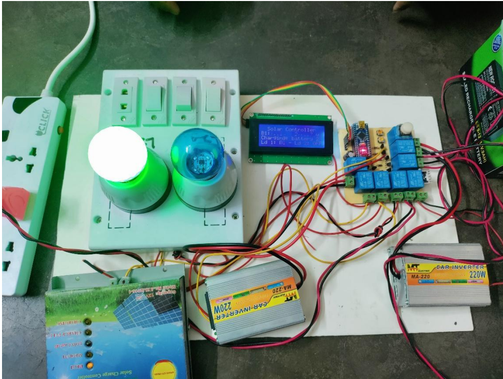
Figure 52: Load 1 is powered by the main battery and load 2 (large loads) is turned off
