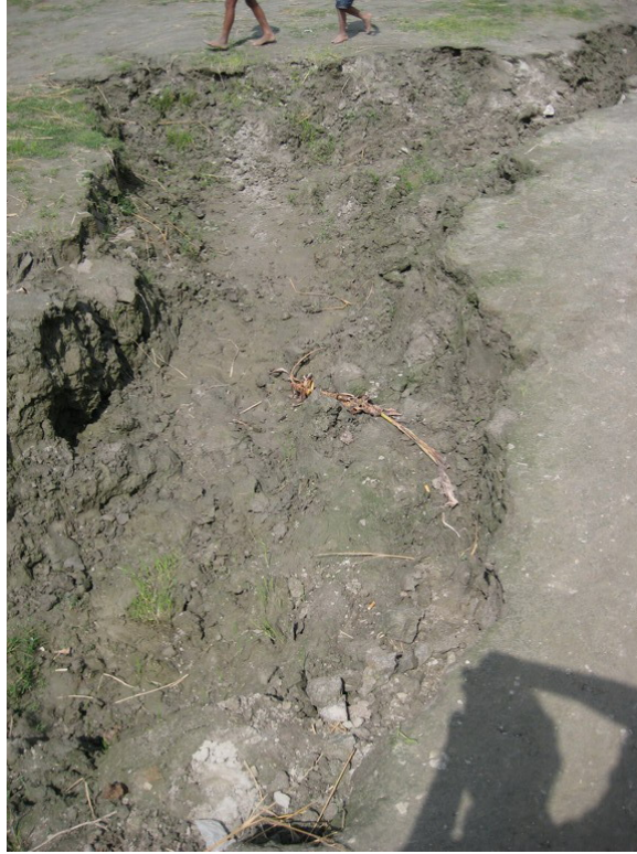
Photo 4.1: Rain cut in a raised community shelter in Sirajganj
