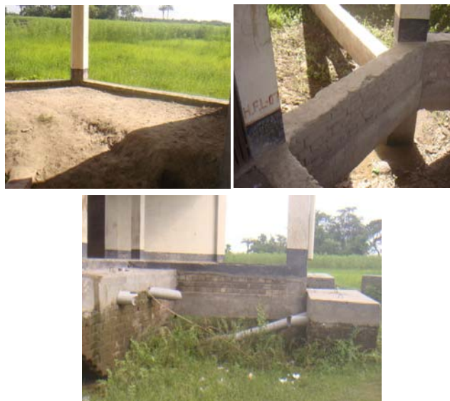
Photo 5.3: Improperly stabilized earthen plinth of Saadipur High School (above). Sewer lines get exposed after the flood (below).
