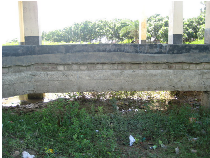
Photo 4.5: Erosion of basement soil by the 2007 flood
