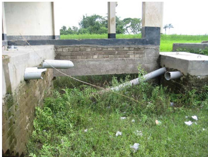
Photo 4.6: Pipes damaged by the 2007 flood
