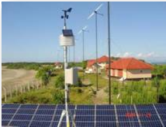
Figure 3.4: Wind-Solar Hybrid System at St. Martin's Island
