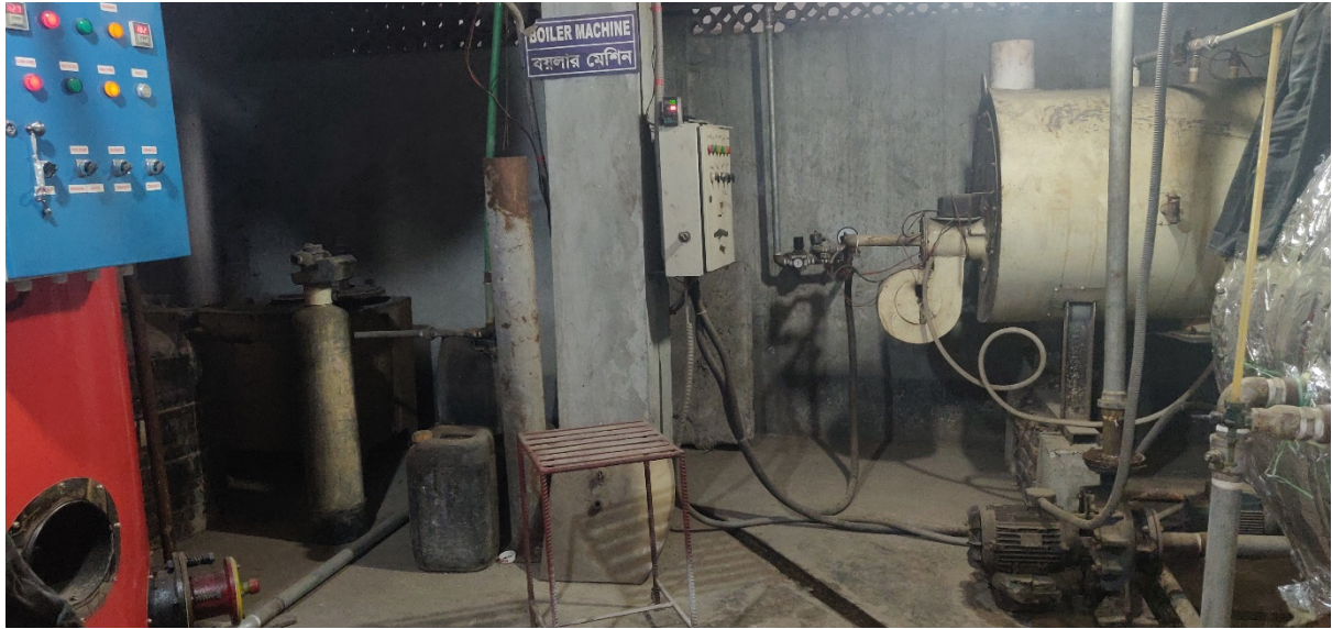
Picture-5: Boiler Machine of Chemical industry.
