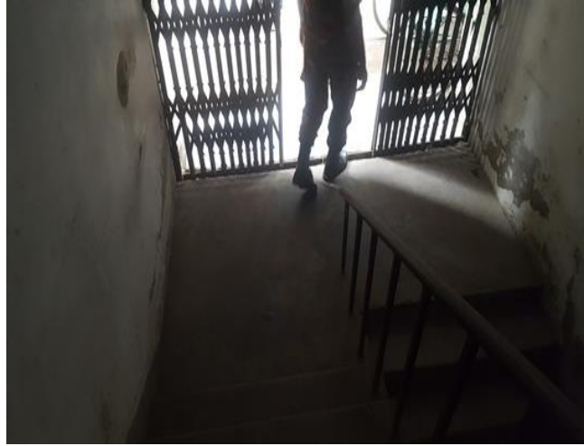
Picture 24: Medona Tower fire escape directly open outside
