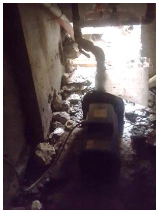
Picture 15: Normal water pump at High tower building
