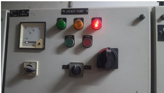
Picture 13: Jockey Pump control
