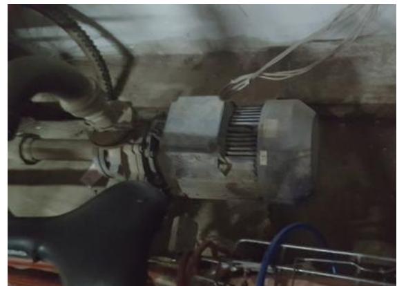
Picture 16: Normal water pump at Aqua tower
