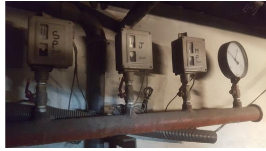
Picture 10: Water pressure gauge
