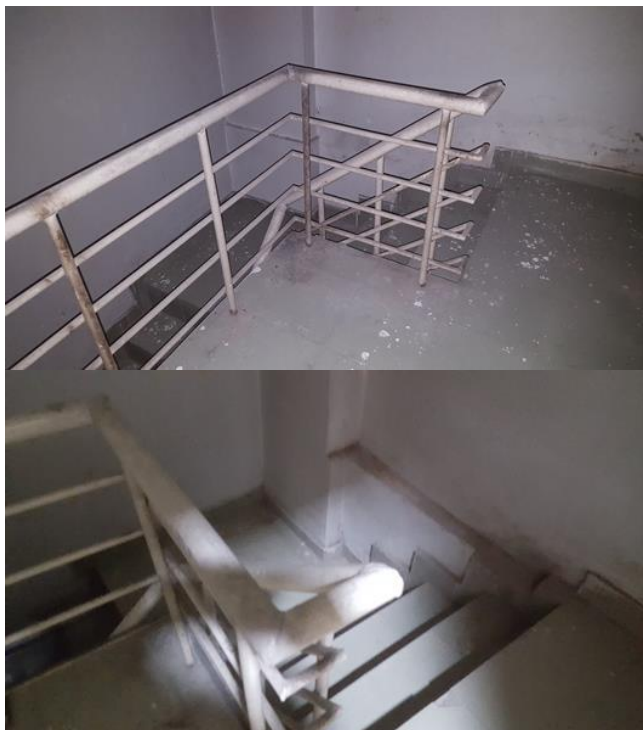
Picture 17: No light at fire escape stairs at JR Casero
