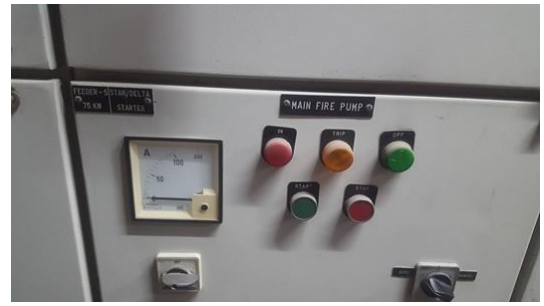
Picture 12: Main fire pump control
