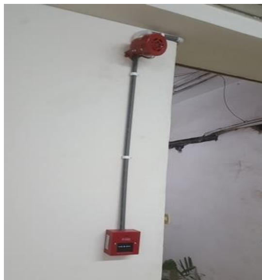
Picture 30: Fire alarm at High Tower
