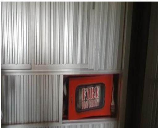
Picture 25: Riser location was inside the room
