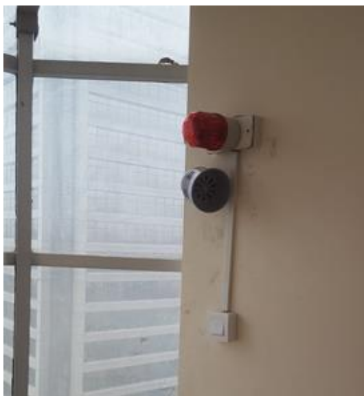
Picture 29: Fire alarm at Haque Tower
