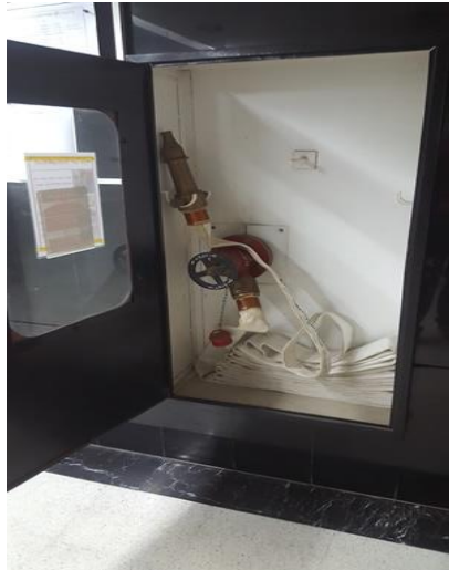
Picture 27: Riser at Civil Engineers Building
