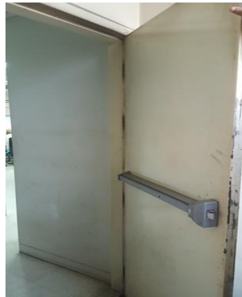
Picture 22: Fire rated doors at Civil Engineers Bhaban
