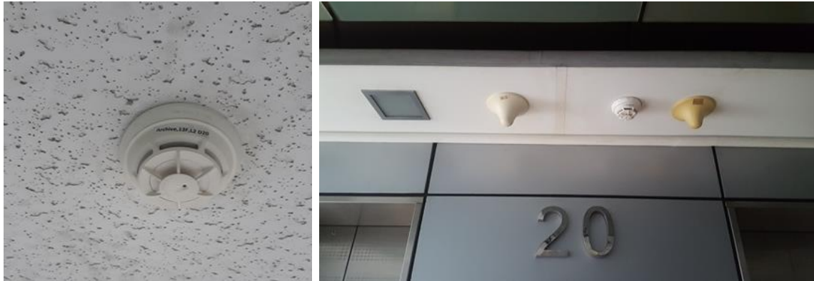
Picture 31: Multidetector system at Civil Engineers Bhaban
