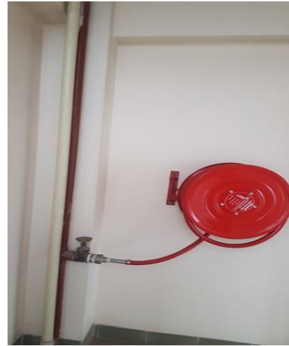
Picture 28: Riser at Haque Tower
