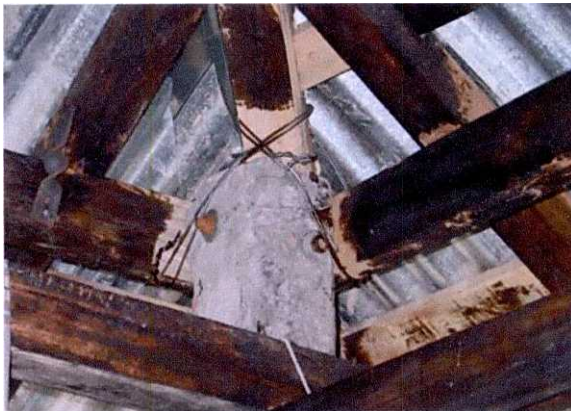
Metal angles, pegs and wires are used for joints. Jute or nylon ropes are not used as it decays in weather.
