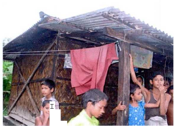
Cross bracings of wall frames are used outside on the shorter length of walls.
