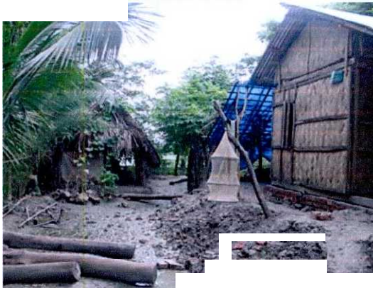
No cross bracing used, wooden frame with vertical and horizontal members used.
