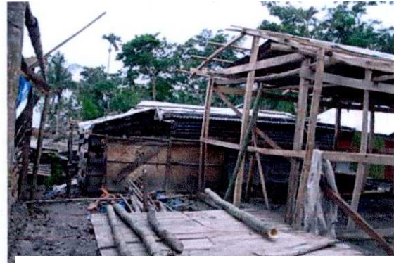
Wood, bamboo, betel nut trunk etc are used in frame according to ability, iron pegs are used in joints.
