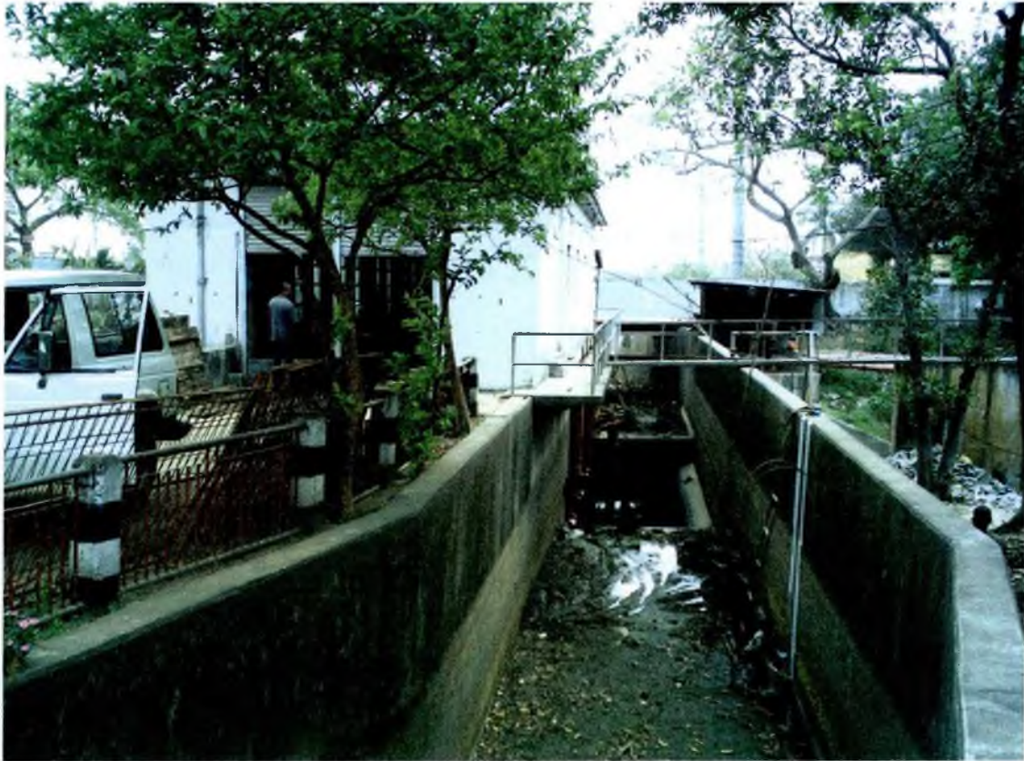
Photo 7.1: Existing Pump Station of DND Area, Shiddirgonj, Demra.
