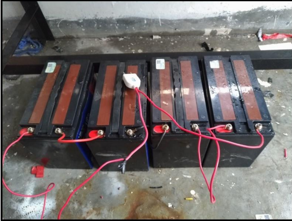
Fig (3.14): Sealed lead acid batteries in series connection
