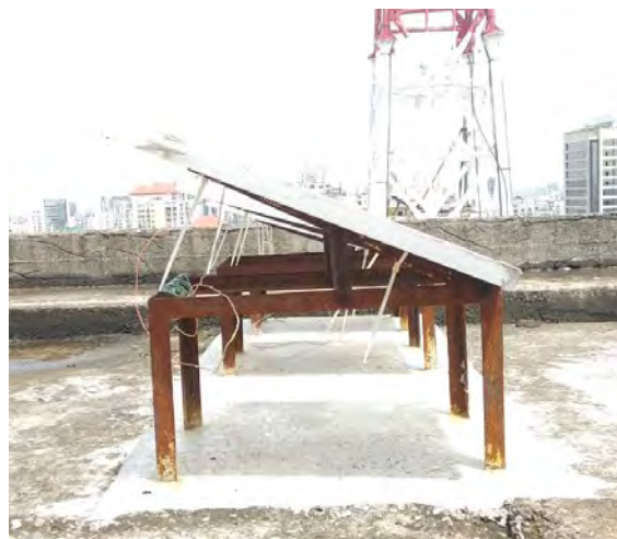
Figure 3.2: Mono crystalline module tied to the iron frame facing south
