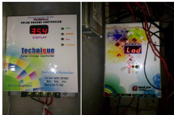
Figure 6: Solar charge controller for solar panel (left) and for wheelchair (right) [1]
