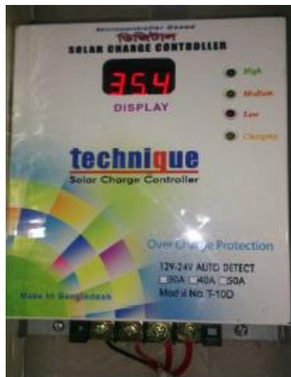
Figure 26: Solar Panels and Solar Charge Controller
