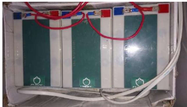
Figure 4: Battery set of the original wheelchair [1]
