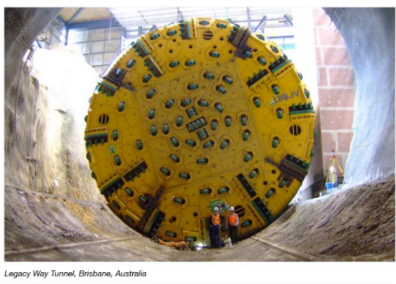
Legacy Way Tunnel, Brisbane, Australia
