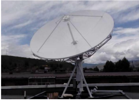
Figure 3.6(a): Parabolic Antenna
