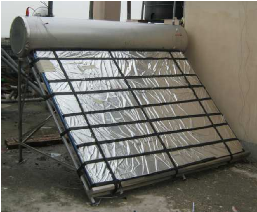
Fig. 3.1: Hot water storage tank insulation with foam and aluminum foil [1].
