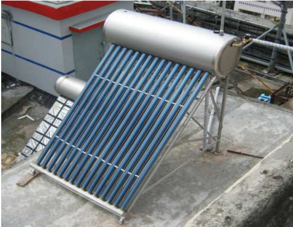
Fig. 2.1: Solar Water Heater installed on the roof of BRAC University [2].
