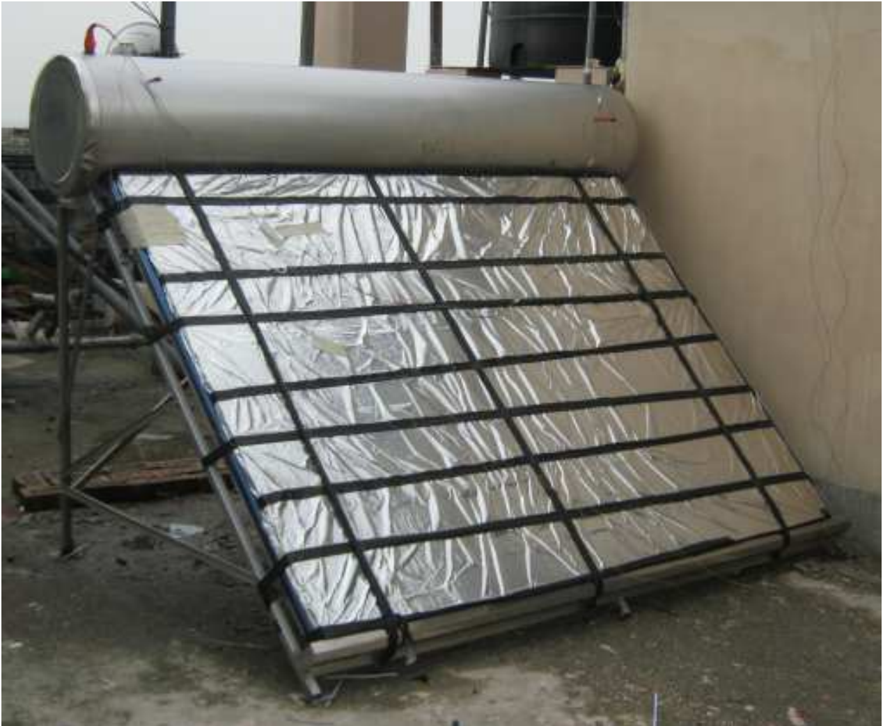
Fig. 2.5: 300-liter solar water heater with insulated collector on the roof top of BRAC University [1].
