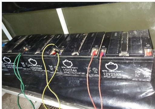
12V 25Ah batteries connected in series
